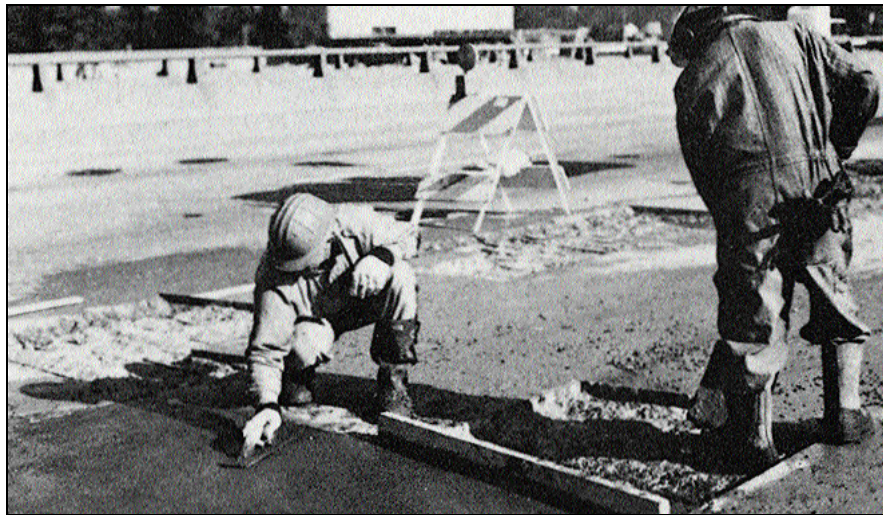
A magnesia-phosphate cement is being used to patch a highway. Its rapid-setting and rapid-hardening properties minimize the disruption of traffic.
